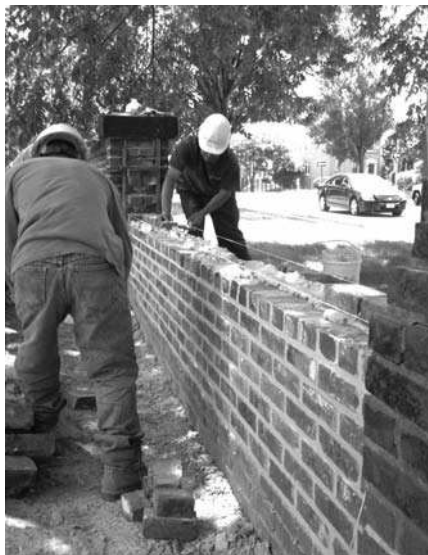
Brickworkers from Pointing Plus filling in the car-sized hole in the 17th Street Wall.
