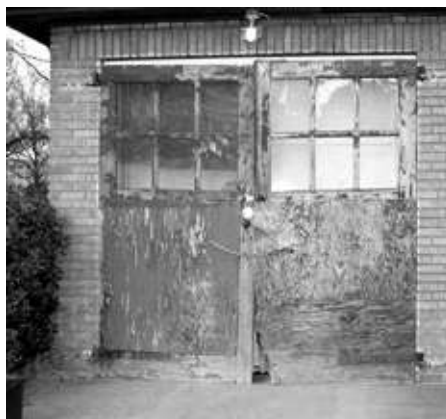
Garage doors to be replaced.
